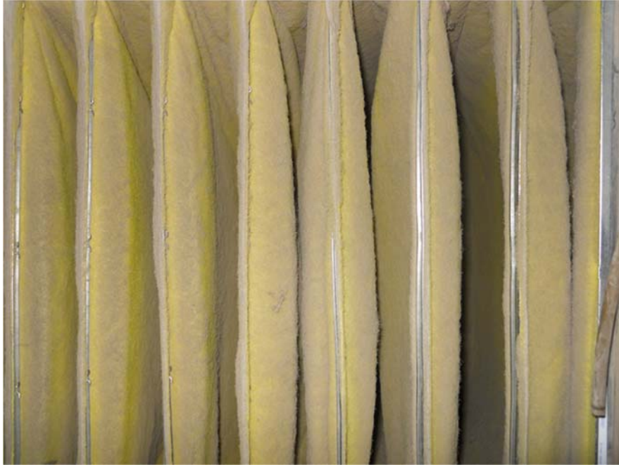
Bag Filters in AHU
