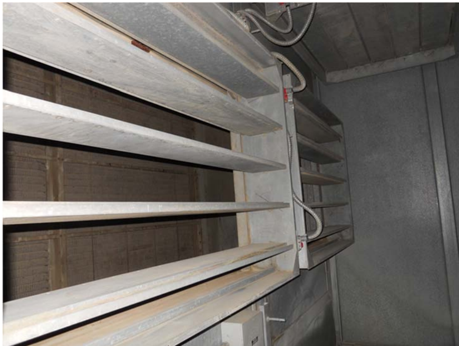
Mesh Pre Filters in AHU
